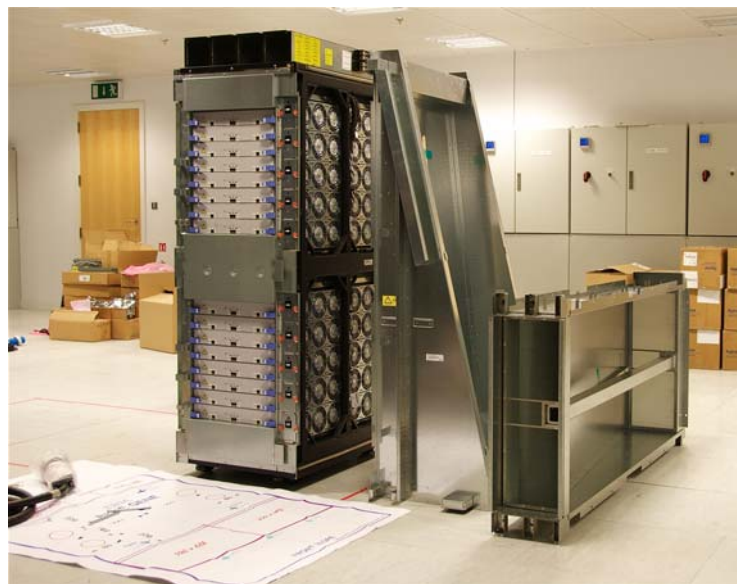
BlueGene /L under construction
